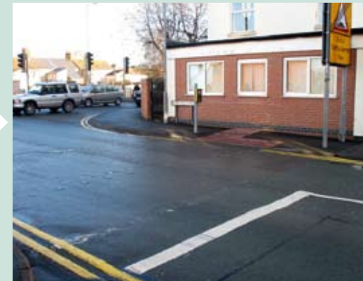
Improved pedestrian facilities at the junction of Jephson Road and Burton Road.
